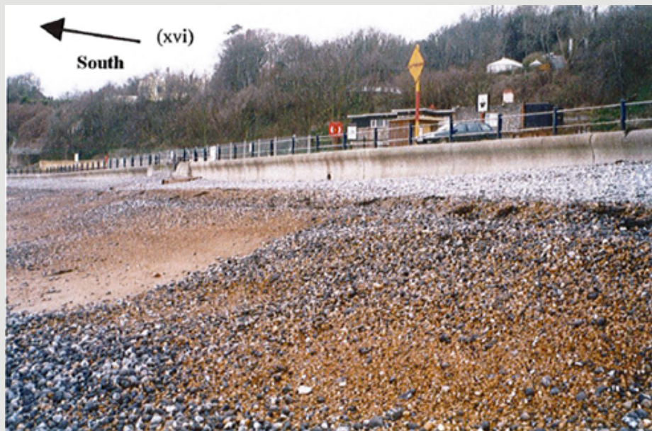
(xvi) At the north end of the beach this sea wall in 1998, built to protect housing behind it.
