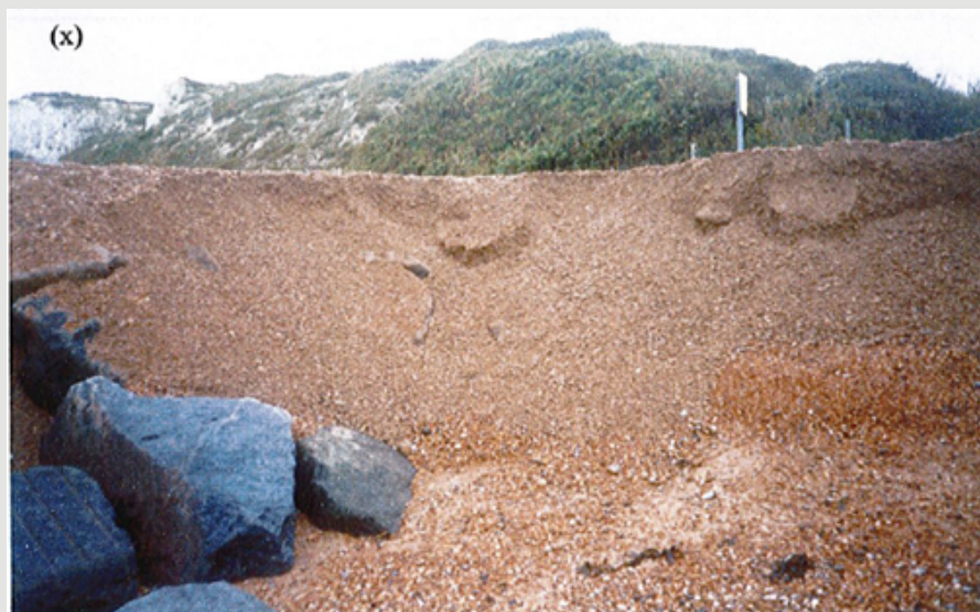
(x) Evidence of recent collapse of the shingle ridge is shown here. This ridge is so unstable that it collapses beneath gentle pressure from a foot.
