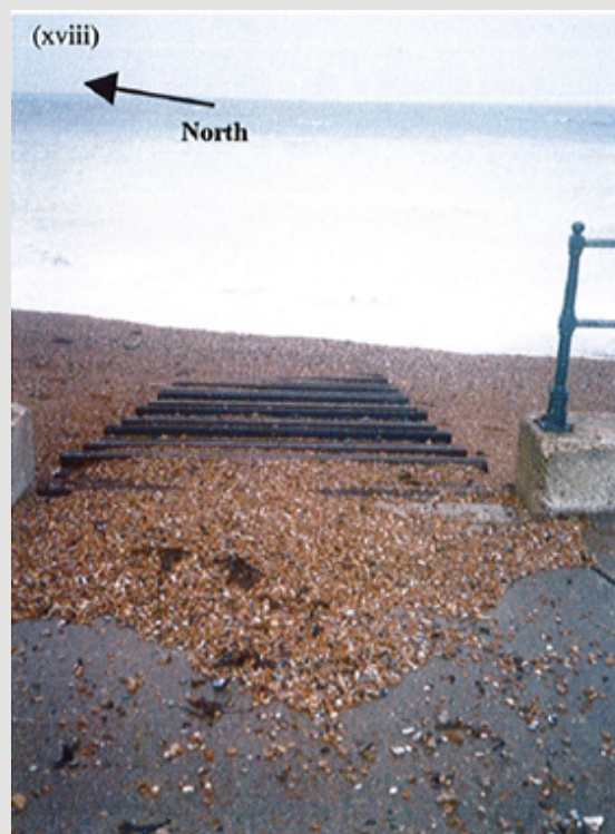
(xviii) The boat ramp at the north end of the beach was built in 1995. Photographed here in September 2000, it has almost been completely buried by shingle from the south.
