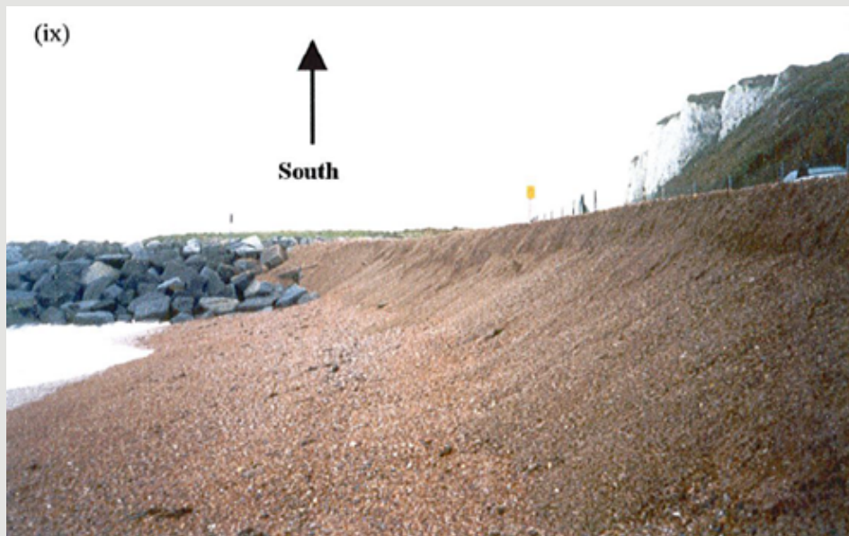
(ix) An extremely steep and unstably shingle ridge (approximately 2.5m high) has developed at the top of the beach. The steepness is caused by repeated undercutting.
