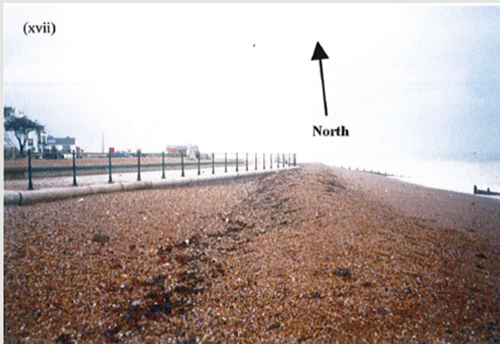
(xvii) This is the same sea wall (from a different perspective) in August 2000. The height of the shingle against the wall has risen about 1m. The shingle has come from the Oldstairs Bay end of the beach.
